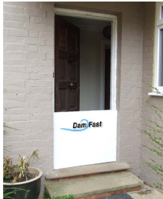
Flood gate in place
